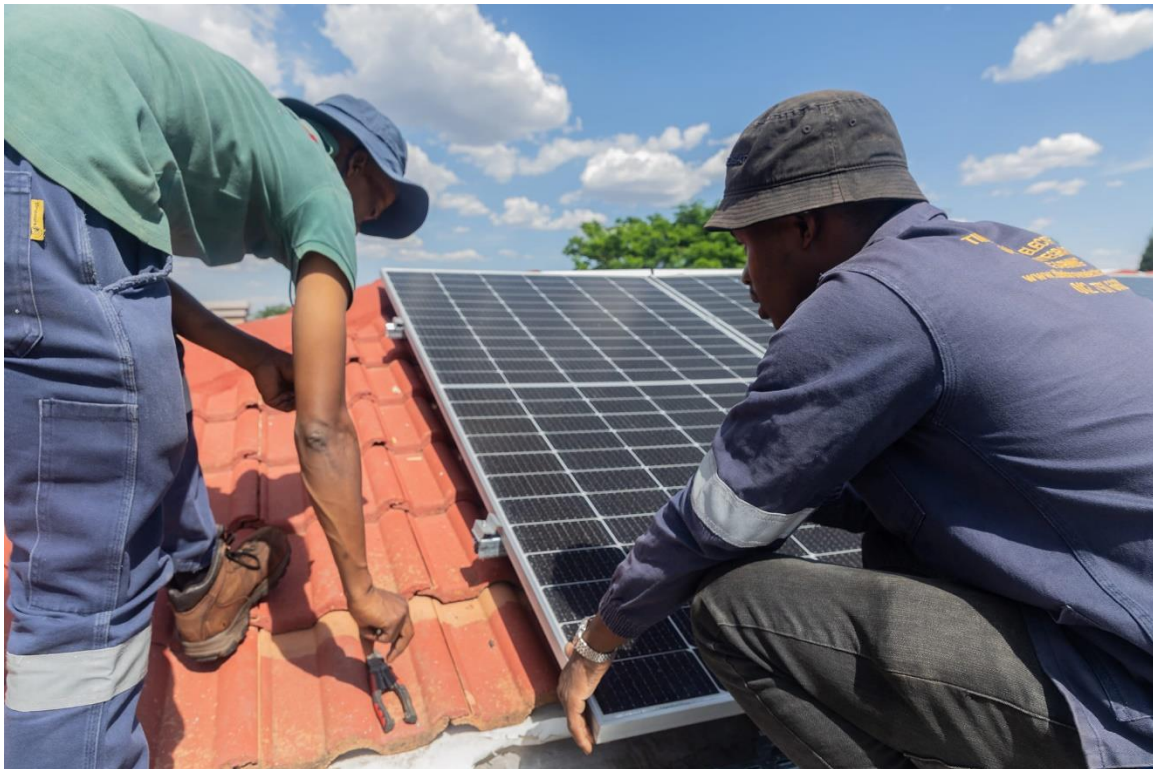
Caption: Energy transition programme beneficiaries install solar panels in a South African community.
